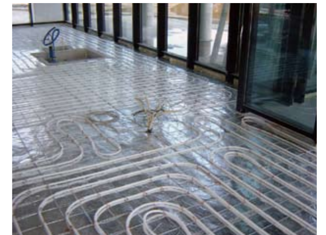
Floor heating on ground floor
